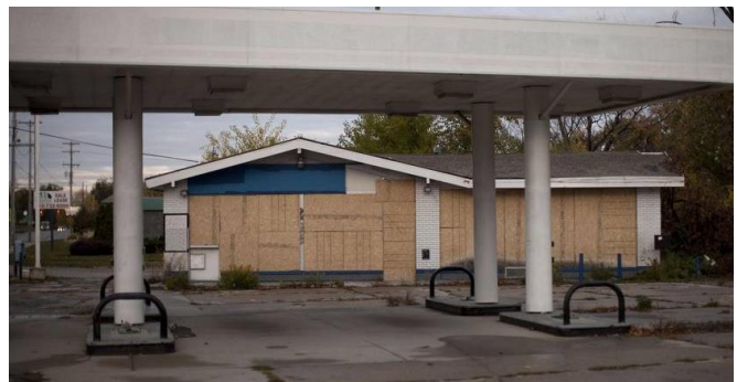
High remediation costs already deter developers from investing in former gasoline retailer sites; these properties often remain vacant for many years.
